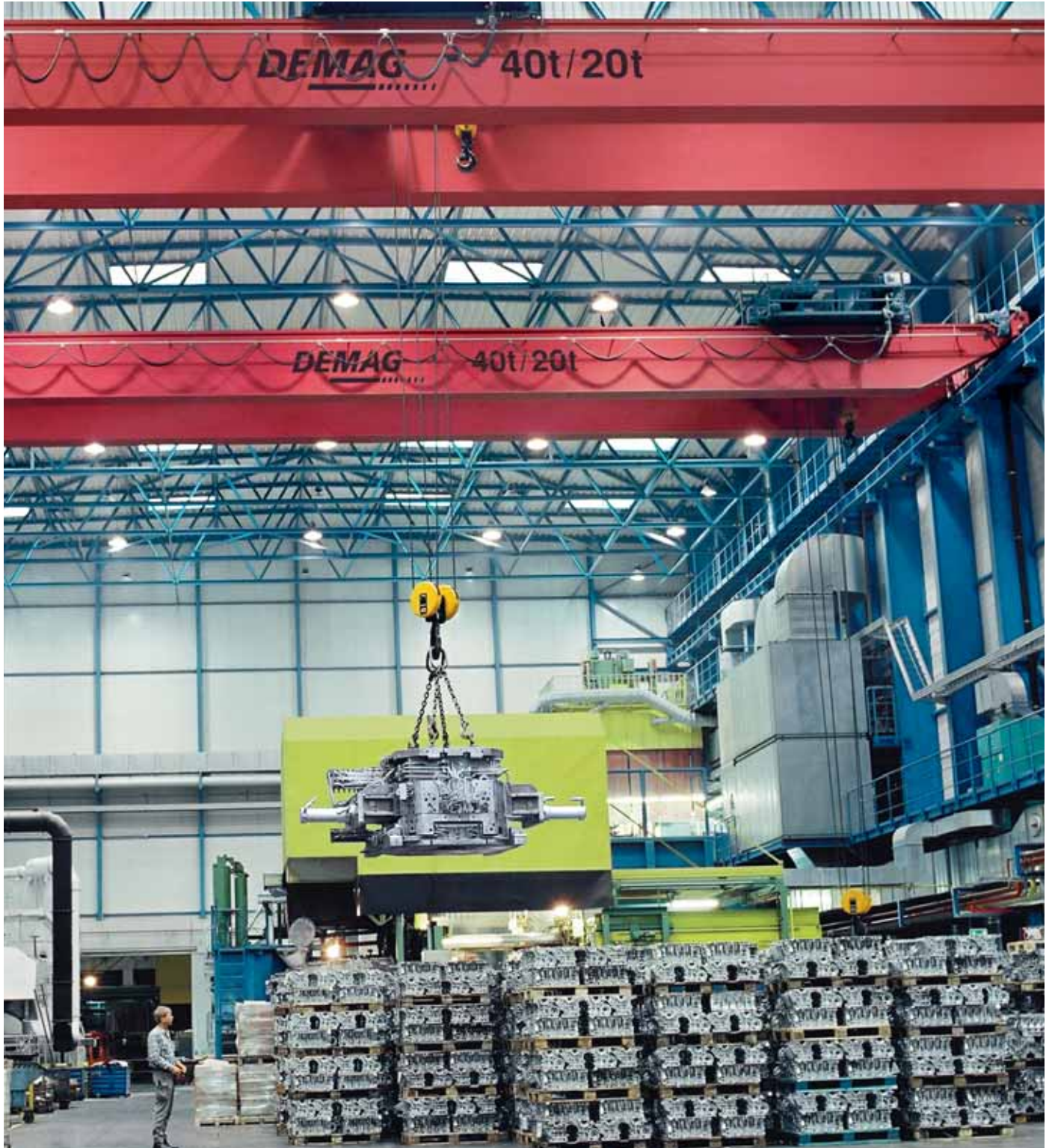
Double girder overhead traveling crane with tandem end trucks for transporting and turning engine blocks
